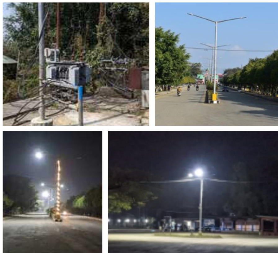
Photograph Plate 8: Heavy Duty Electric Transformer for power supply and LED-based street lights to use during night installed in the Manipur University
